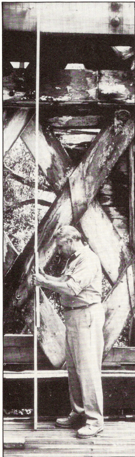
This 1971 photo shows Milton Graton at work measuring inside the bridge for the placement of the laminated arch.
